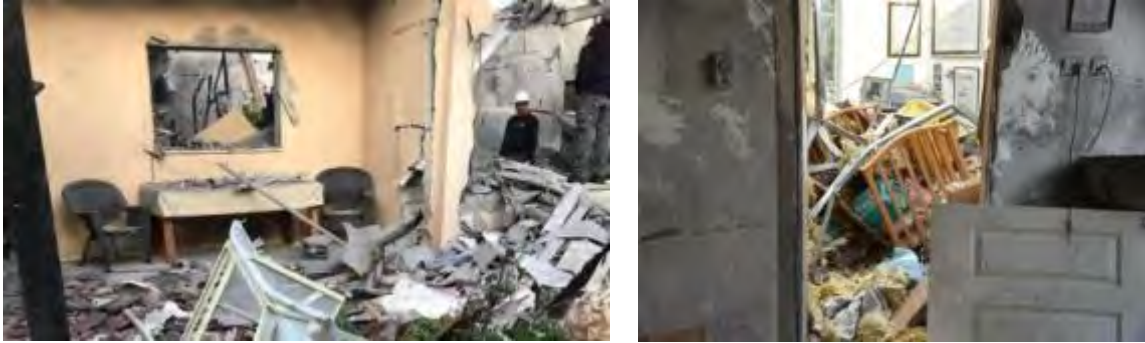
Damage caused by the rocket to a house in the village of Mishmeret (Right: Israel Police. Left: Israel Fire and Rescue Services, March 25, 2019)
