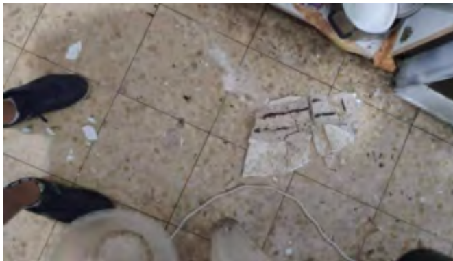
Damage to an unoccupied building in Sderot (Palinfo Twitter account, August 25, 2019)
